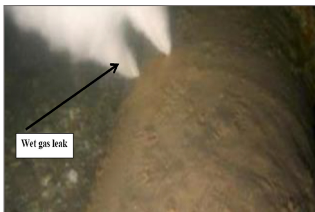
Fig. 9 Photo of TLC pipeline failure (under water) caused by the condensation of water vapor on the top of the pipe in presence of \text{CO}_2 and volatile organic acids (acetic and formic acid). (Ajayi, 2015).
